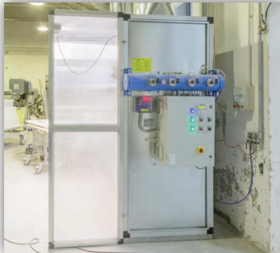
QUADRO CON INVERTER ELECTRIC PANEL WITH INVERTER
